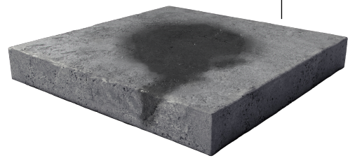
Untreated Concrete, Showing Chloride Induced Corrosion
